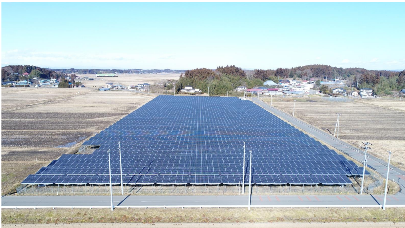
Vitec Tome Solar Power Plant
